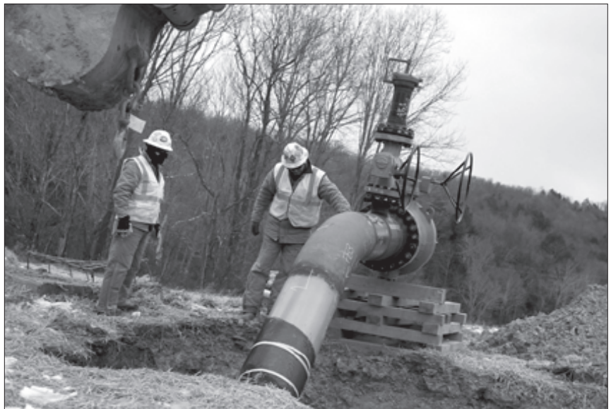
Workers inspect a natural gas valve at a fracking site in Pennsylvania, USA. While advances in fracking technology are set to make the US the world's top oil producer, the overall global outlook for future energy supply is uncertain.
