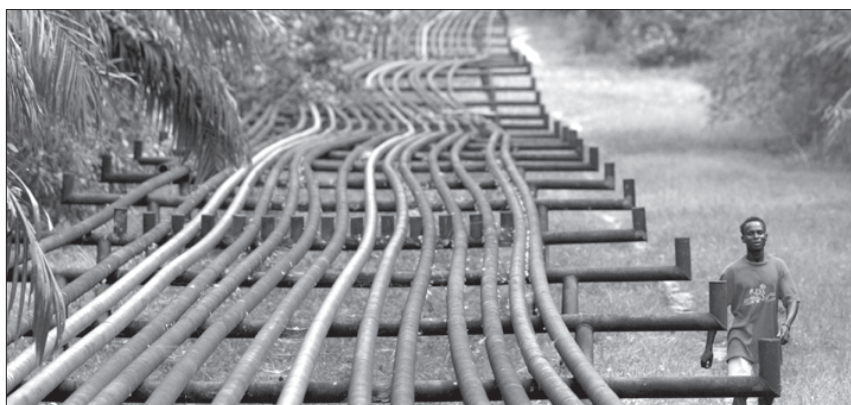
Oil pipelines running through Obrikom, Nigeria. Oil-dependent Nigeria is one of the African sovereign bond issuers which are reliant on one major export product to generate foreign exchange.
