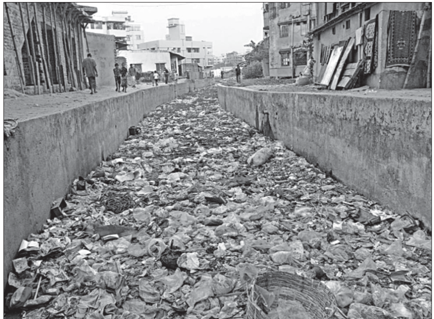
City canals play a vital role in running off rainwater during the rainy season but most of Dhaka’s canals are clogged up by dumped waste.
