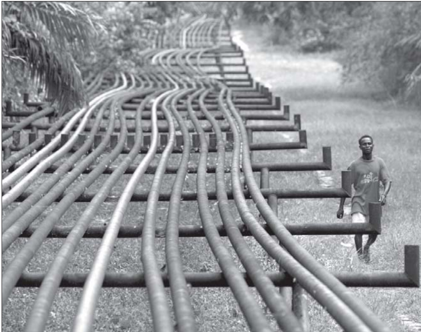
Oil pipelines snaking across a part of the Niger Delta. Nigeria is one of the largest oil producers in Africa and the sixth largest in the world.
