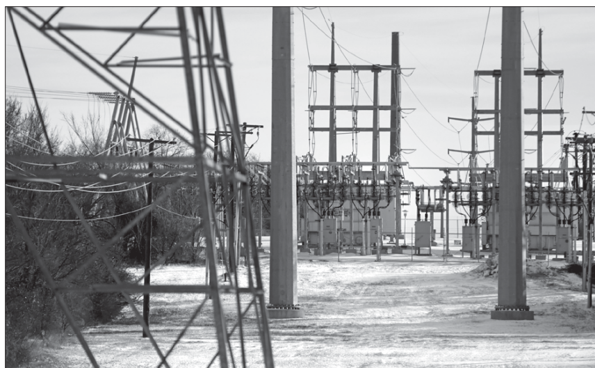
Transmission towers and power lines leading to a substation after a snowstorm in Fort Worth, Texas, in February. The entire Texas power grid came within minutes of a collapse at one point during the cold wave.
